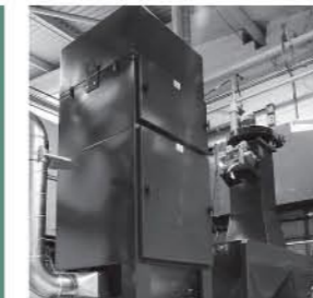
Materials handling extraction system. Fabric shaker and reverse jet cartridge filter
