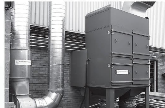
Chemicals processing exhaust system with fume control equipment
